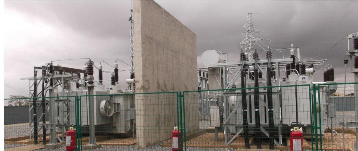
Rehabilitation and Expansion of the Luanda Electricity Network Project, Angola
